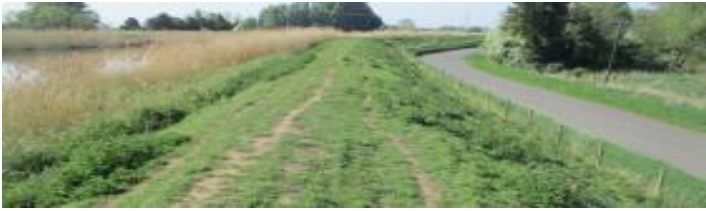
Figure 2: Visible sheep rutting on embankment crest (credit: Georgie-Lee Heeley)
