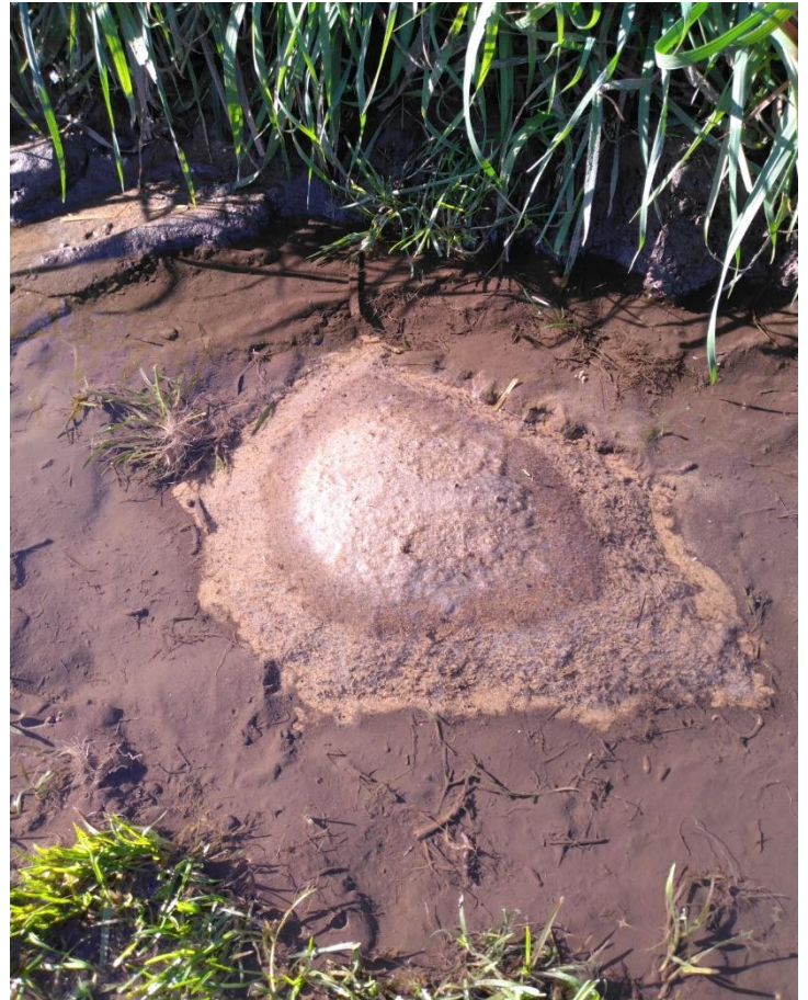
Figure 5: Sandboil – Montjean-sur-Loire levee (Source: EPL, February 24, 2026)
