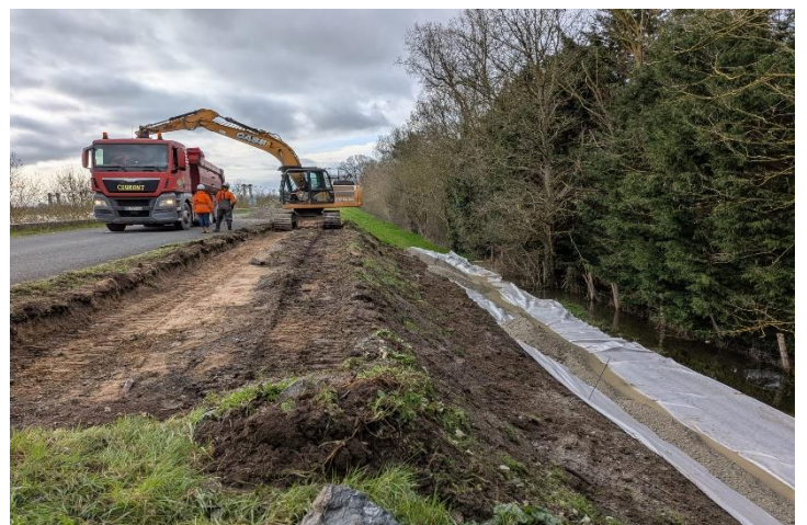
Figure 6: Emergency works on an area of material-laden leakage – Saint-Georges-sur-Loire levee (Source: EPL, February 22, 2026)
