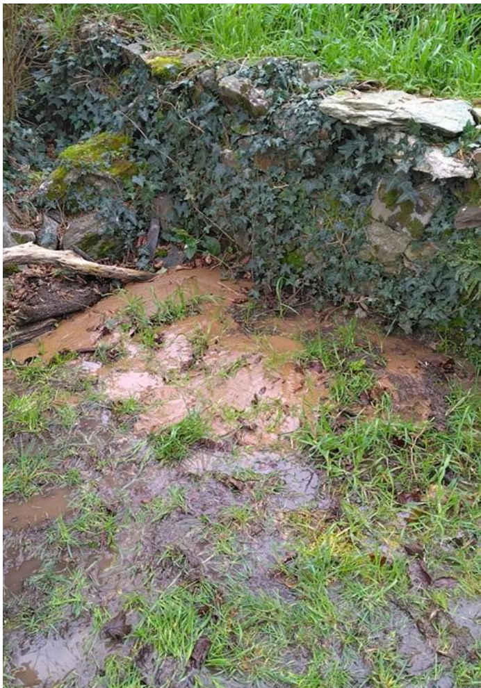
Figure 4: Sediment-laden seepage – Saint-Georges-sur-Loire levee (Source: EPL, February 22, 2026)
