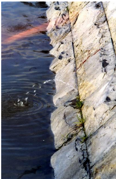
Photo 5.9 A leak through the joints of a masonry revetment, after a flood. This can lead to erosion behind the masonry (Arles, France).
