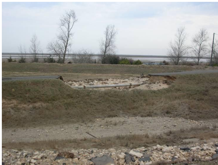
Photo 5.8 Breach of a coastal levee (Vendee, France) exposing a longitudinal pipe
