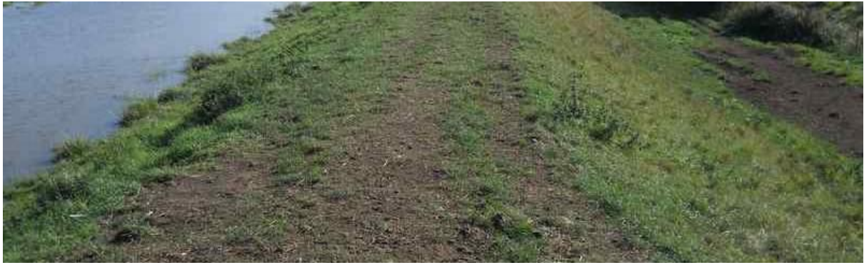
Figure 3.11 Bare soil on the embankment crest
