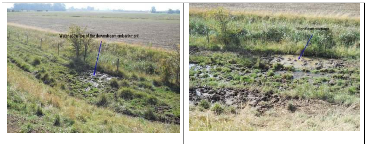
Figure 3.13 Seepage at two locations along the embankment in Winterringham
