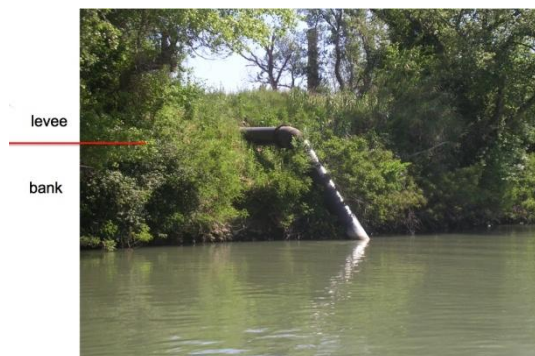
Photo 5.4 A pipe crossing through and across the water side of a levee (Rhône River)
