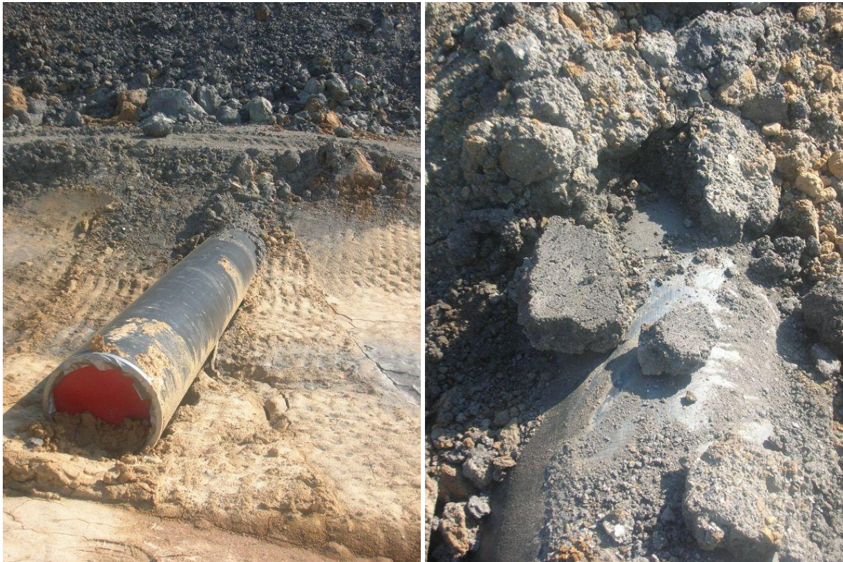
Figure set 5.6A pipe crossing at the base of a levee (Dresden)
