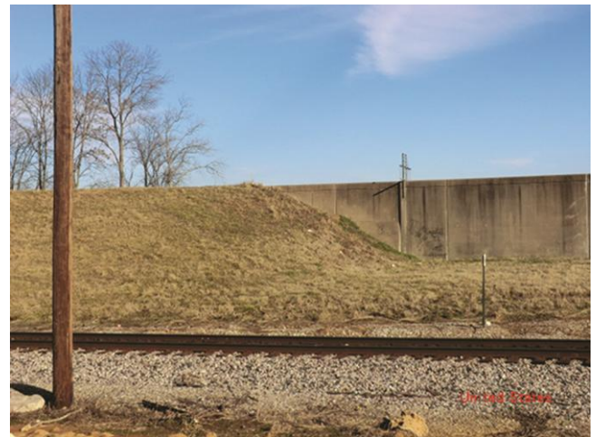
Photo 5.15 transition between a levee and a flood wall in Cape Girardeau, Missouri, USA (source ILH, USACE)
