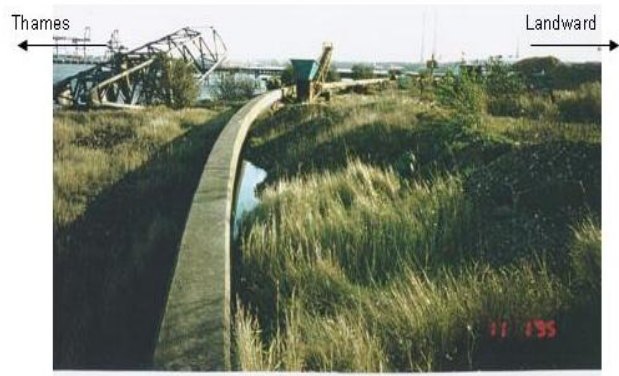
Photo 5.12 Concrete wall on top of levee defences in the River Thames Estuary (UK).
