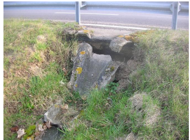
Photo 5.17 Runoff water channel on a levee slope. Transition between grass cover and stonework.
