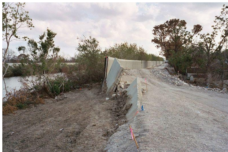
Photo 5.13 New Orleans, London Avenue Canal (Photo: www.online-utility.org )
