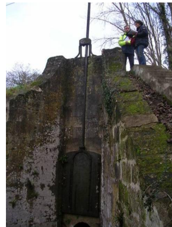
Photo 5.5 A gate control at the end of a culvert passing through a levee (River Loire)
