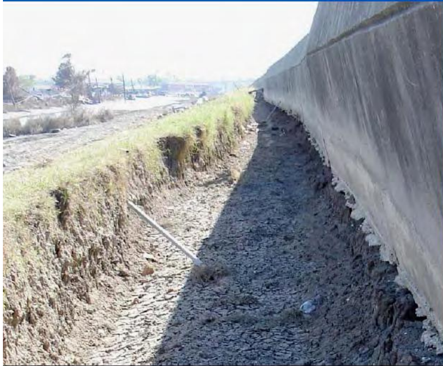
Figure: Scour and Erosion on the Protected Side of the IHNC Adjacent to the 9th Ward in the Vicinity of the South Breach
