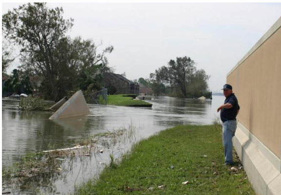
Photo 5.11 17 th Street Canal levee breach (Hurricane Katrina, New Orleans, USA)
