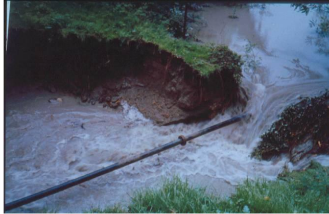
Photo 5.6 Levee breach initiated along a pipe crossing (Rhône River). Photo SNRS.
